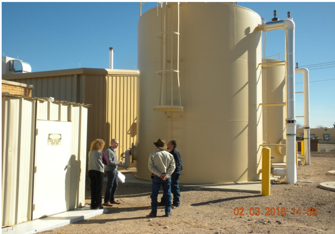
Mr. Mark Purcell (EPA-RPM), Ms. Adrienne Widmer (CLC-Utilities Administrator), and CLC-Utilities Facility Operators, discuss the remedial system operations next to the two 28,000-gallon equalization tanks on the west side of the treatment system building (South view).
