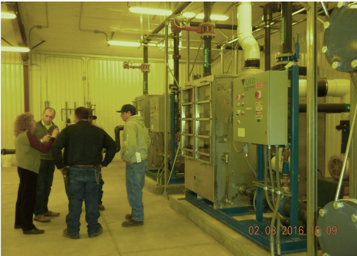
Mr. Mark Purcell (EPA-RPM), Ms. Adrienne Widmer (CLC-Utilities Administrator), and CLC-Utilities Facility Operators, discuss the remedial system operations in the main room next to the two parallel stacked-tray air strippers (South view).
