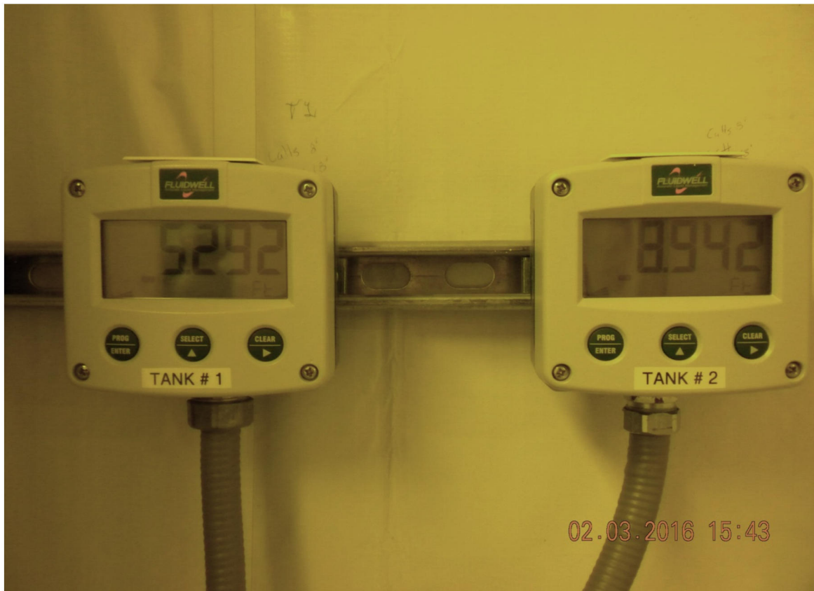
LCD monitors at the operator interface terminal indicate the water levels in the two 28,000-gallon equalization tanks (extracted/raw water and treated/finished water) (South view).
