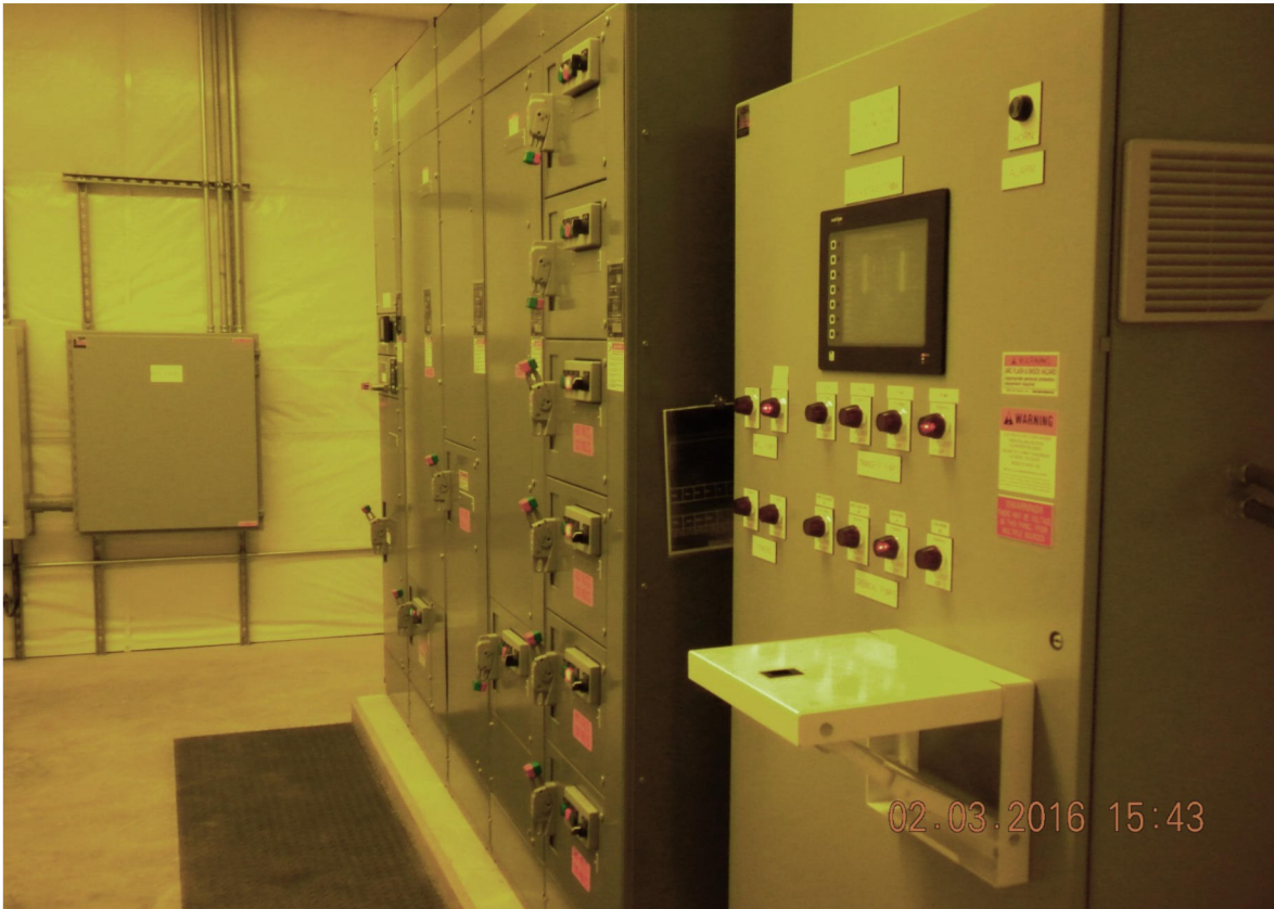
Water treatment facility process control panel inside the treatment system control room (East view).
