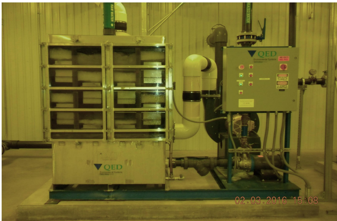
Close-up view of a QED Environmental Systems single stacked-tray air stripper and control panel, with water transfer pump and air blower that forces air through the stacked trays of untreated/raw water in the air stripper to remove VOCs (West view).
