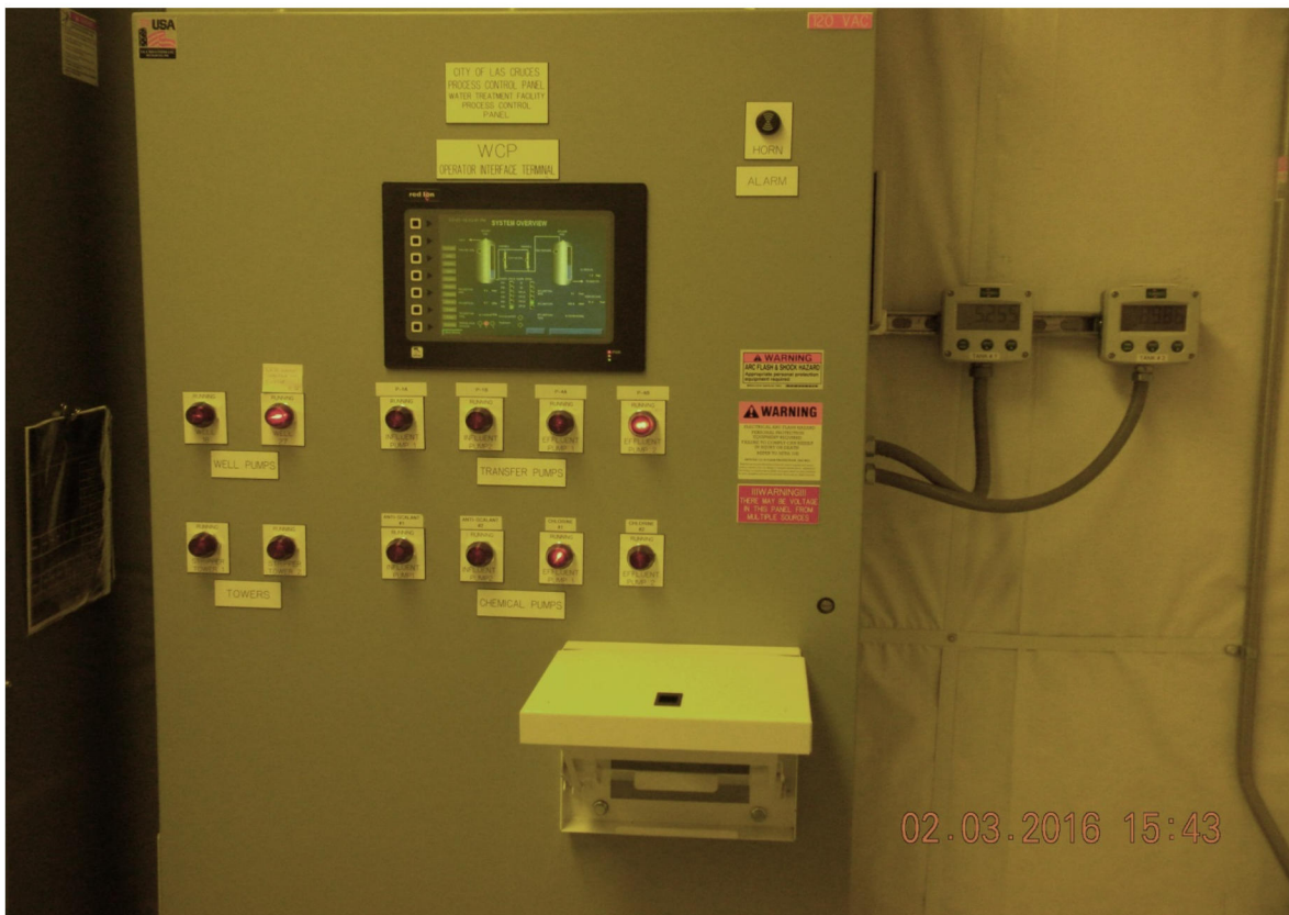
Close-up view of the water treatment facility process control panel and operator interface terminal (South view).
