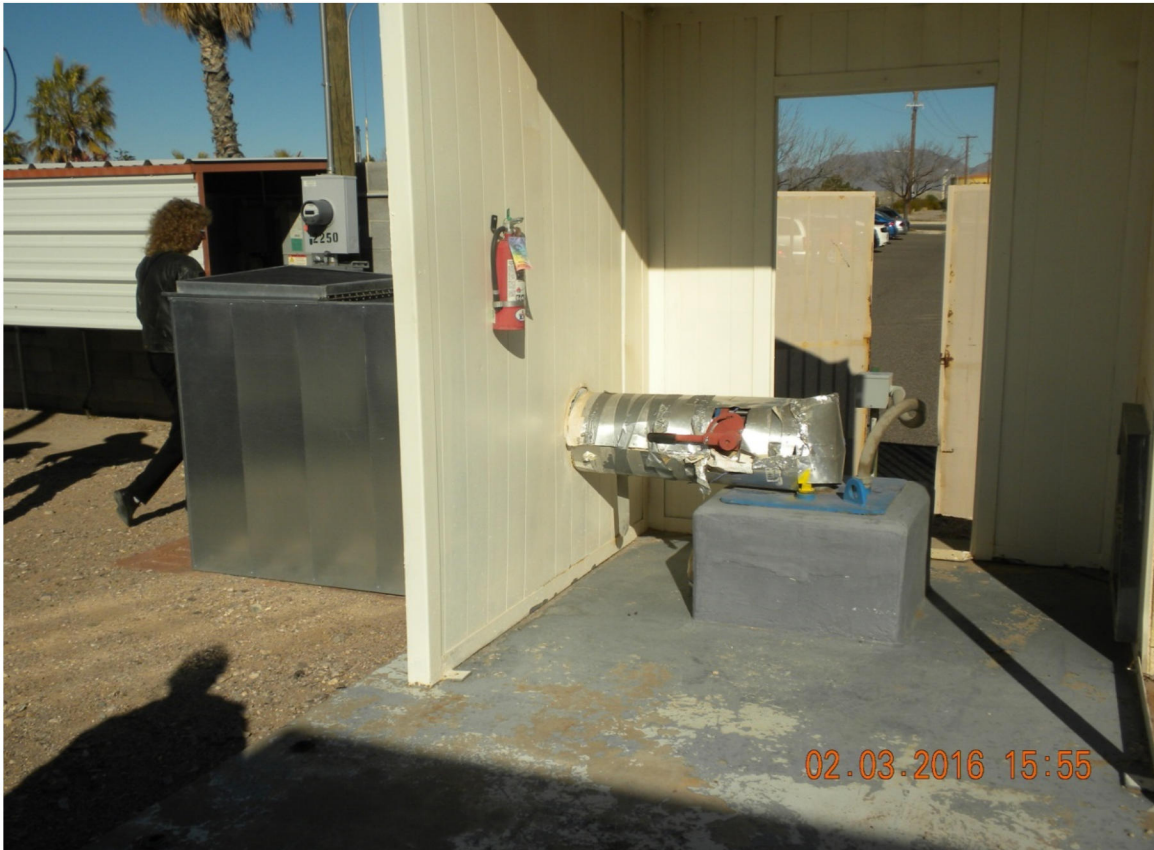
CLC Well 27 and well house enclosure located west of Walnut Street on the south side of East Griggs Avenue (East view).
